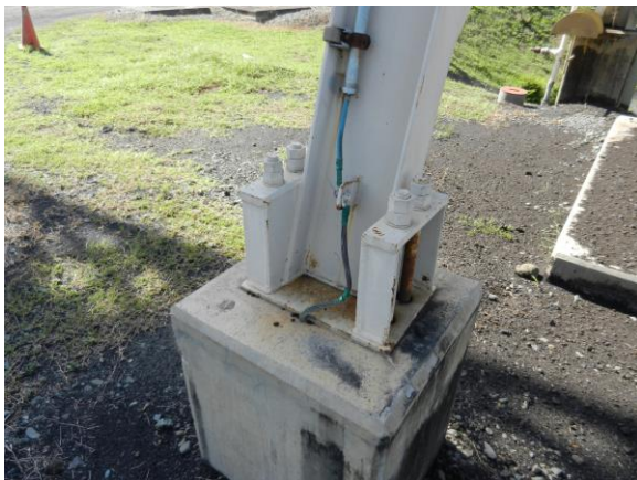
5. Concrete Encased Electrode (CEE)
