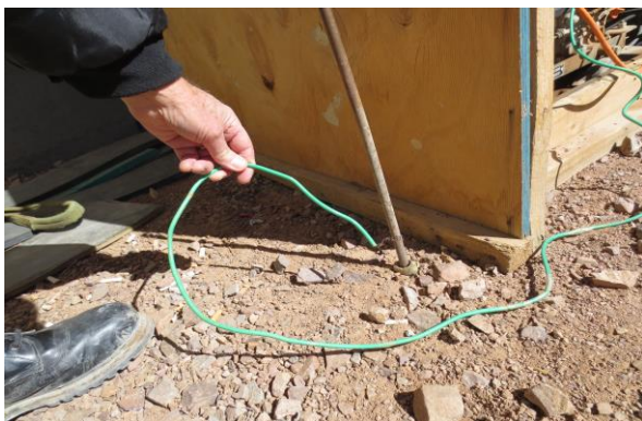
3. Inadequate Bonding Connector
