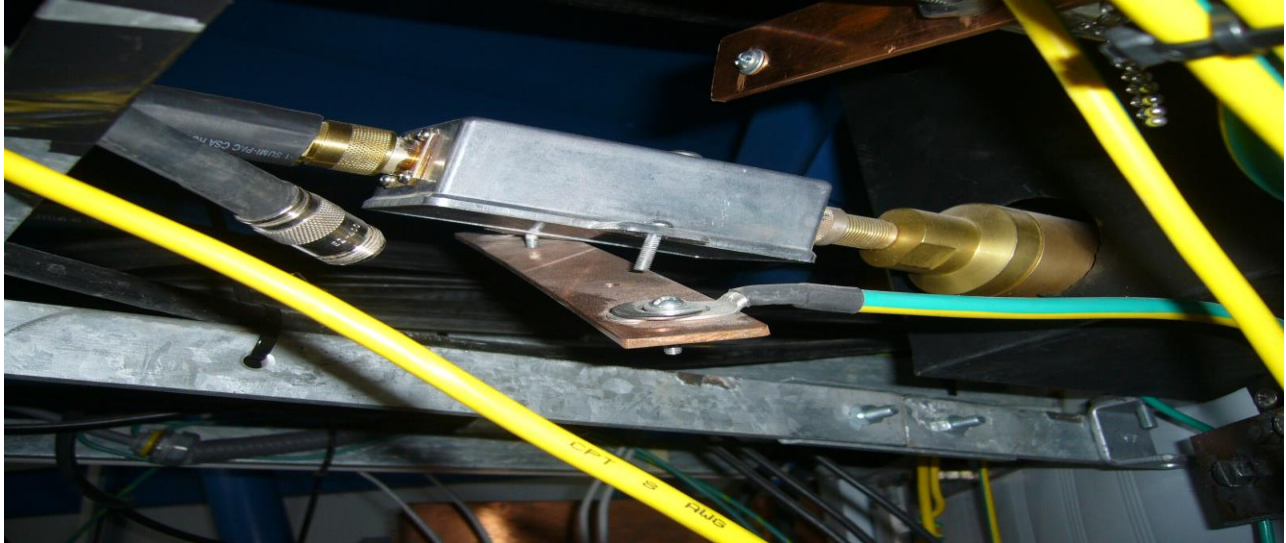
9. Coaxial Cable Signal Lines Showing Improper Installation
